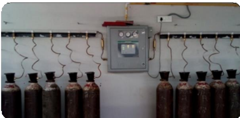
(Hospital Oxygen Gas System)
